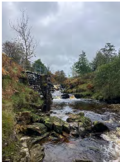
Figure 16: Photo of UU infrastructure and reinforced bankside on New Water
